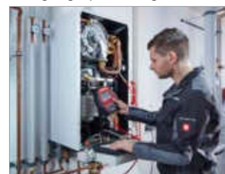
Testing of gas pressure regulators
